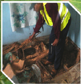
Coptotermes gestroi (Causing Structural damage)
